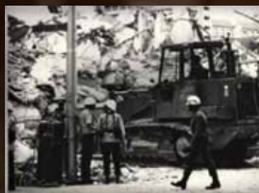
Engineers assisted in rescue efforts of victims trapped under the rubble of Singapore's worst post-war disaster.
