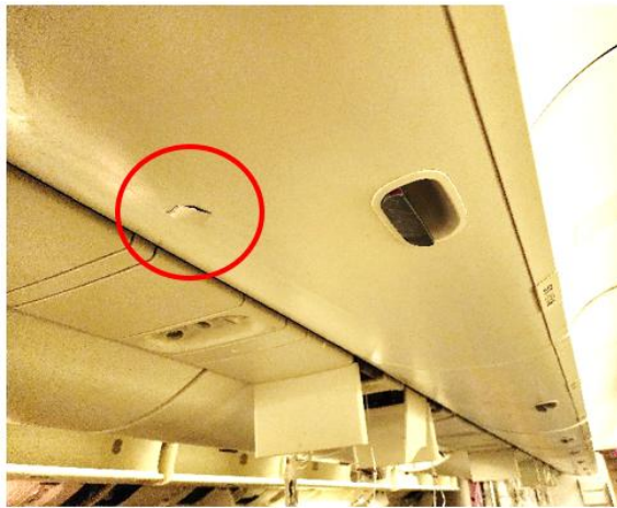
Figure 6: Punctured overhead bin
