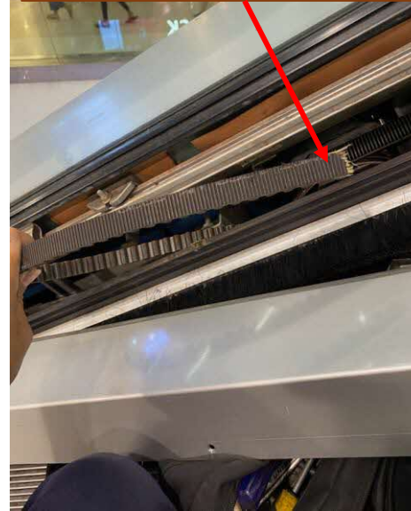
Broken Handrail Drive Belt
