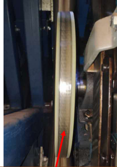
Worn out Handrail Sheave.
