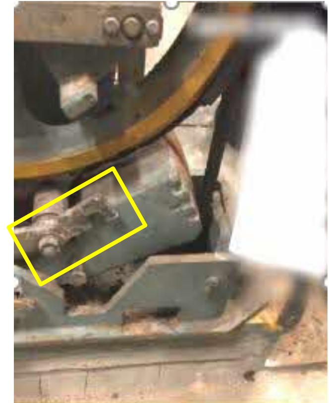
Video – Overspeed Governor with restricted parts, not sufficiently lubricated.
