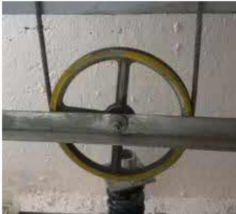
- No Switch installed. - Fixed on Bracket. No Tensioning
