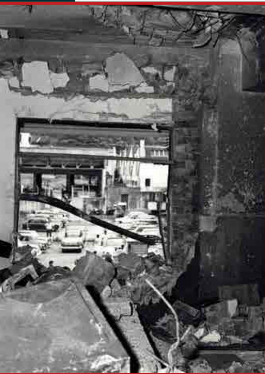
Damage from the bomb explosion at MacDonald House on 10 March 1965. The concrete wall separating the stairway and correspondence room of the Hongkong and Shanghai Bank was blown apart by the bomb, exposing the car park on the other side. Source: The Straits Times © SPH Media Limited. Reprinted with permission.
