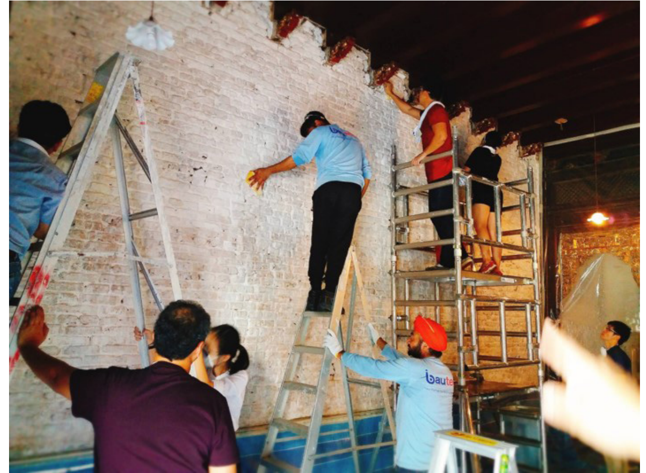
Participants plastering a wall as part of the programme in April 2019 on the technology and use of lime plaster in buildings. © Nikhil Joshi.
