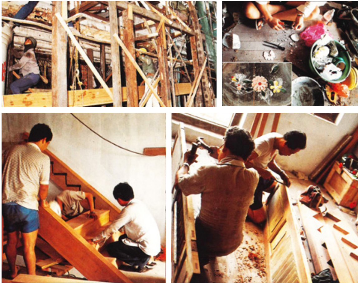
The restoration work of 9 Neil Road as a showcase which took three months to complete showing the replacement of the fascia beam, staircase and remoulding the ornamentation.
