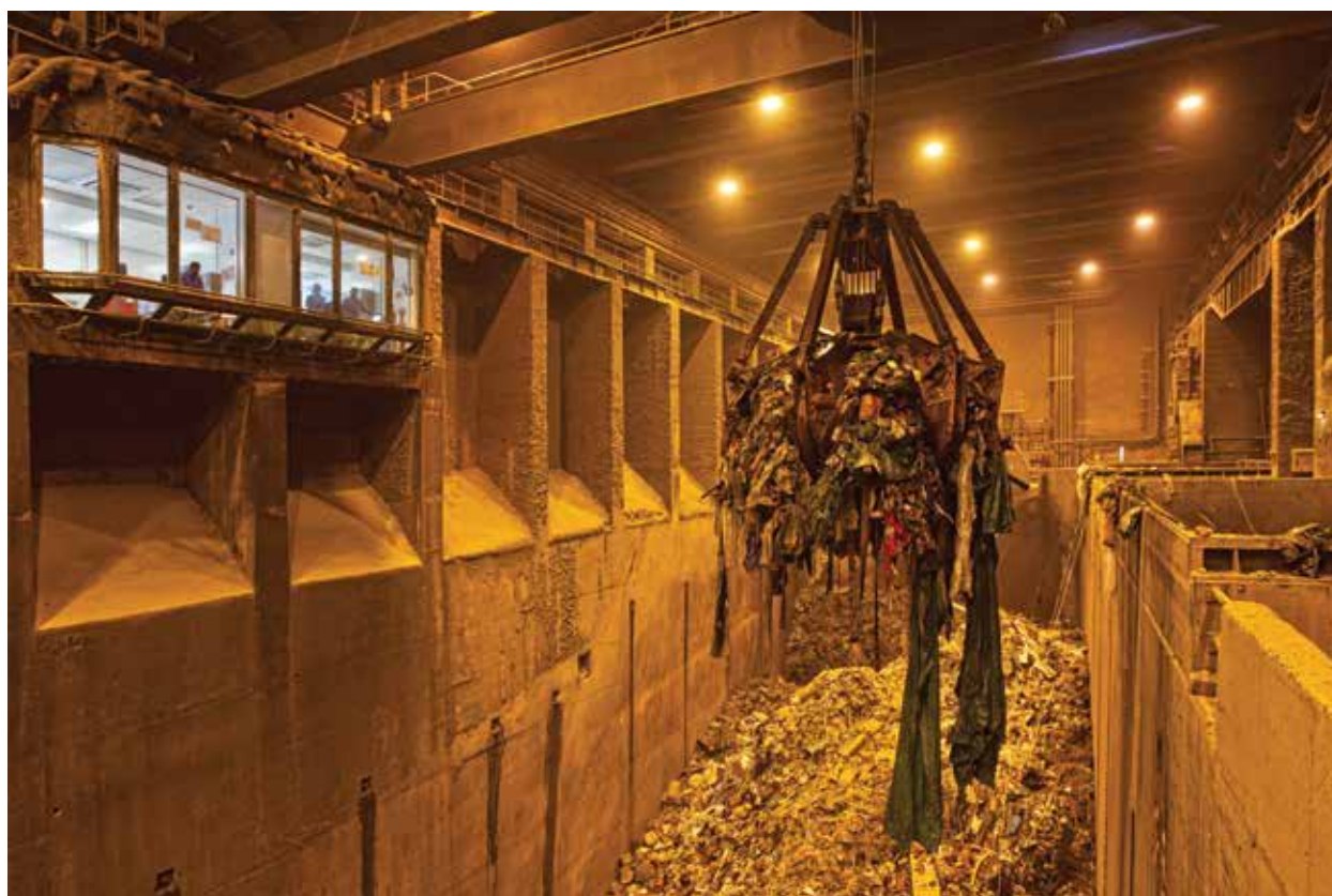
Refuse bunker in Singapore's waste-to-energy incineration plant.
